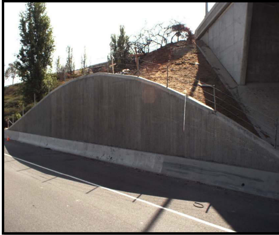
Figure 6.2: An MX8 MTLs system camera image of the automobile accident embankment site on SR 74
