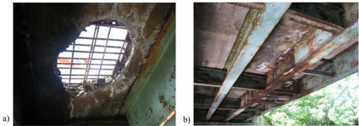
Figure 3.7: a) Hole through the deck, and b) map cracking with heavy efflorescence at the O-03-009 bridge
