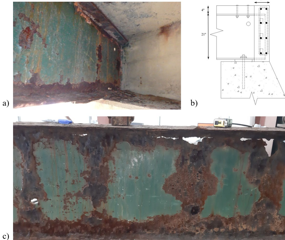
Figure 3.2: (a) In-service configuration, (b) construction details for the support, and (c) web condition at midspan
