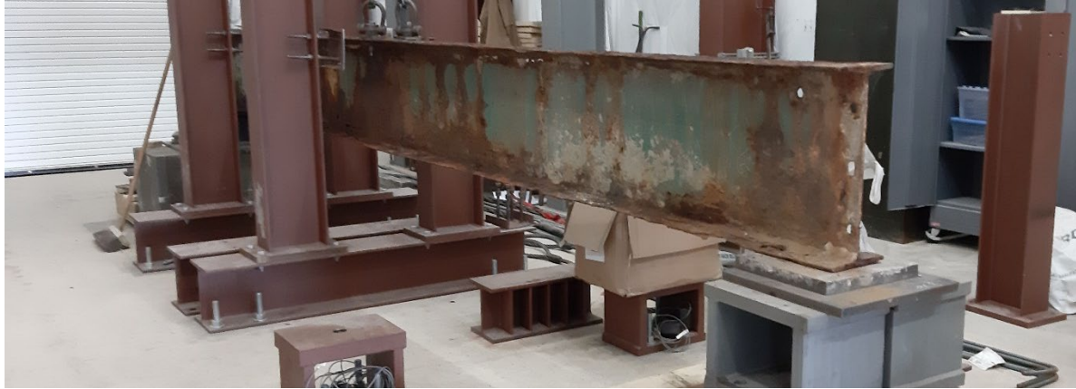
Figure 3.1: Field corroded girder used for the study
