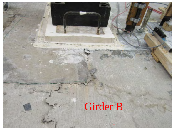
f. LMC Continuous Joint after Testing
