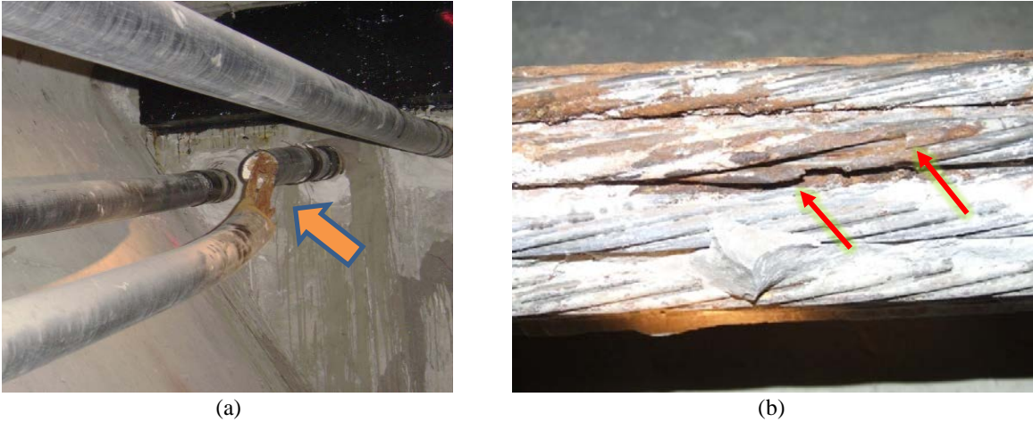
Figure 1. Corrosive Attack on Post-Tensioned Structural Strand: (a) corrosion of individual strand wires ultimately causing an overload failure of the middle external tendon (orange arrow); middle tendon is hanging by the broken wires inside the other half of the duct; (b) section loss in high-strength steel strand, with red arrows showing ends of a fractured wire
