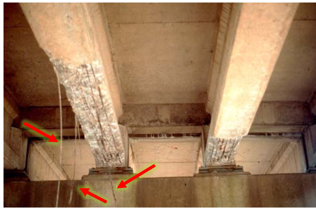
Figure 2. Failure of Corroded Conventional Steel Strands. Some have snapped and now hang down (red arrows) along the bottom of several beams because of leaking bridge deck joints.
