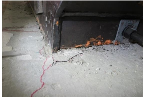
(c) Damage near loading side
