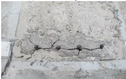
(c) Split cracks near column reinforcement
