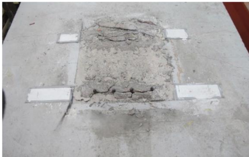
(a) Cracks on top surface
