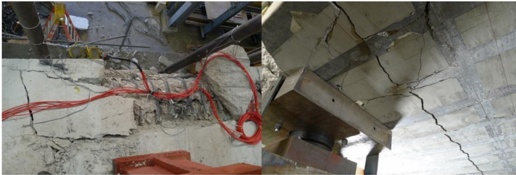
(a) Damage on the top of side face of V-13
