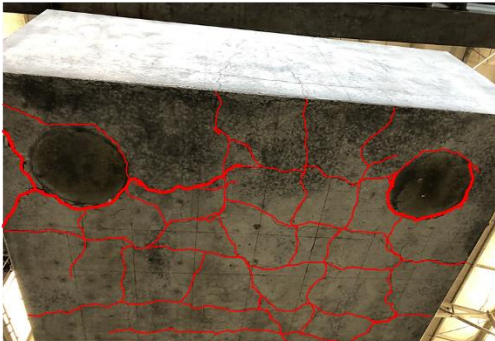
(b) Damage near support side
