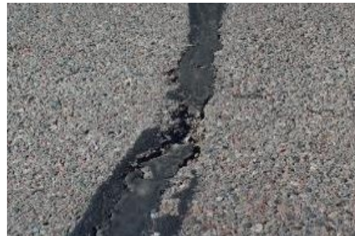
(ii) Pull-out Failure
