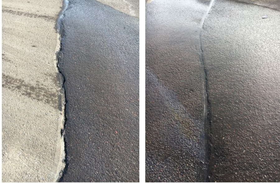
(a) Failed Crack Seal
