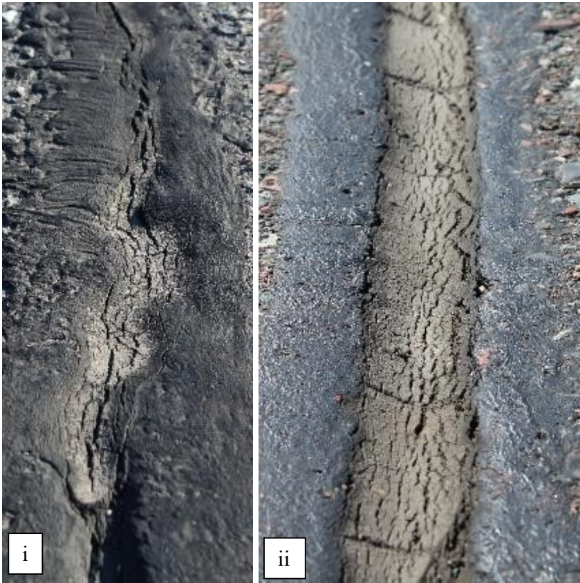
Figure 4.29: (i) Cohesion Failure of Clean-and-Seal Crack (ii) Early Signs of Cohesion Failure on Rout-and-Seal Crack
