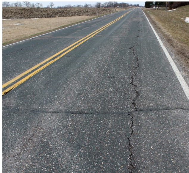
Figure 1.3 Photograph of a Longitudinal Crack
