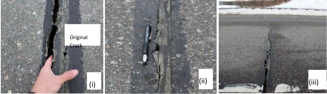
Figure 4.28: Examples of Seal Failures (i) Spalling, (ii) Partial Adhesion Loss, (iii) Full-depth Adhesion Loss.)
