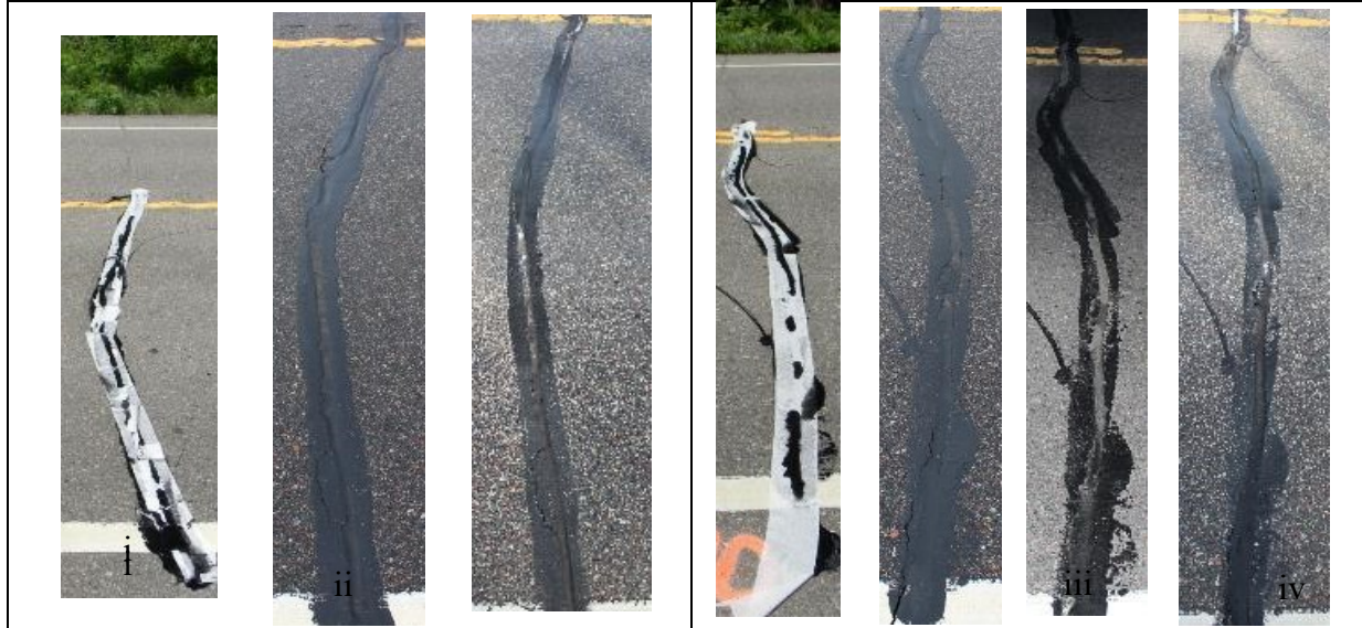
Figure 4.32: Photographic Performance Documentation of Site E. E-1-i Shows Crack E-1 upon being sealed. E-1-ii and E-1-iii show Crack E-1 at the end of its first winter and during the second winter after being sealed. This same sequence of photos follows for cracks E-2, E-3, E-4, E-5, E-6, E-7, E-8, E-9, and E-10. E-10-iv shows the seal performance at the end of the first winter compared to the mid-winter performance presented in E-10-iii.
