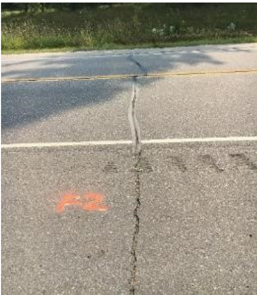
Figure 1.2 Photograph of a Transverse Crack
