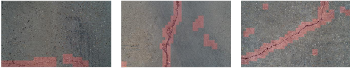
(a) Identified cracks in concrete images
