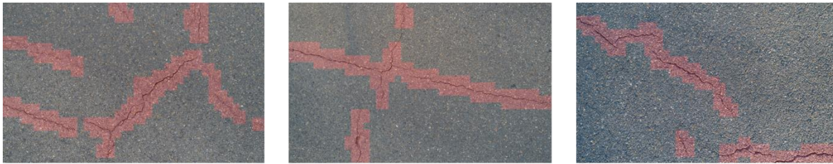
(b) Identified cracks in asphalt pavement images
