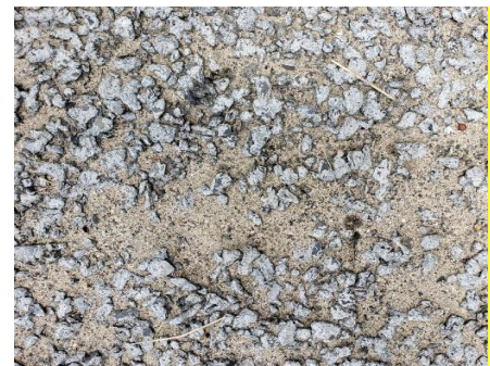
Severe raveling and clogging can occur if not maintained
