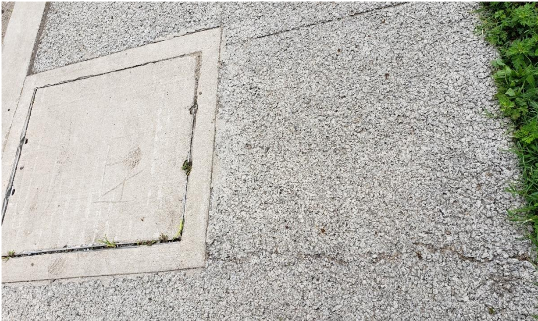
Figure 5. Porous concrete surface showing a crack initiating from the corner of the utility manhole (Location B)
