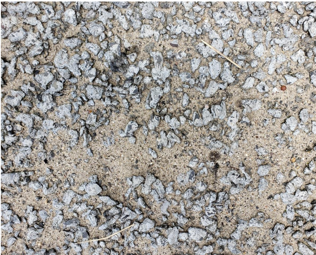
Figure 7. Severe clogging and severe raveling (Location C)
