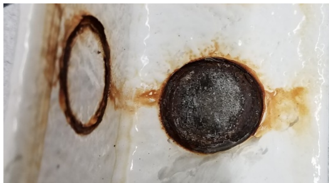
Steel Surface after the pull-off of circular-coating-patch at early stage: Very little corrosion and loss of pull-off strength.
