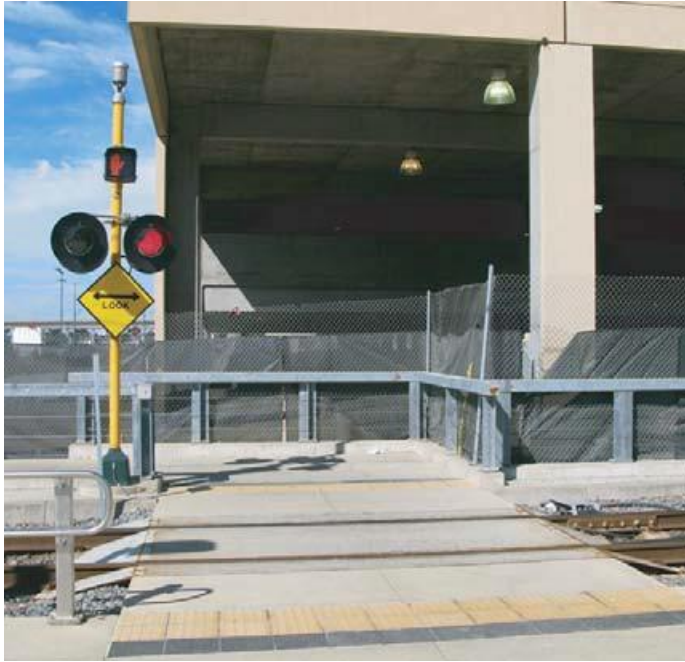
Figure 34. Pedestrian signal with “LOOK” sign and flashing lights, Metro Transit’s Hiawatha line, Minneapolis, MN
