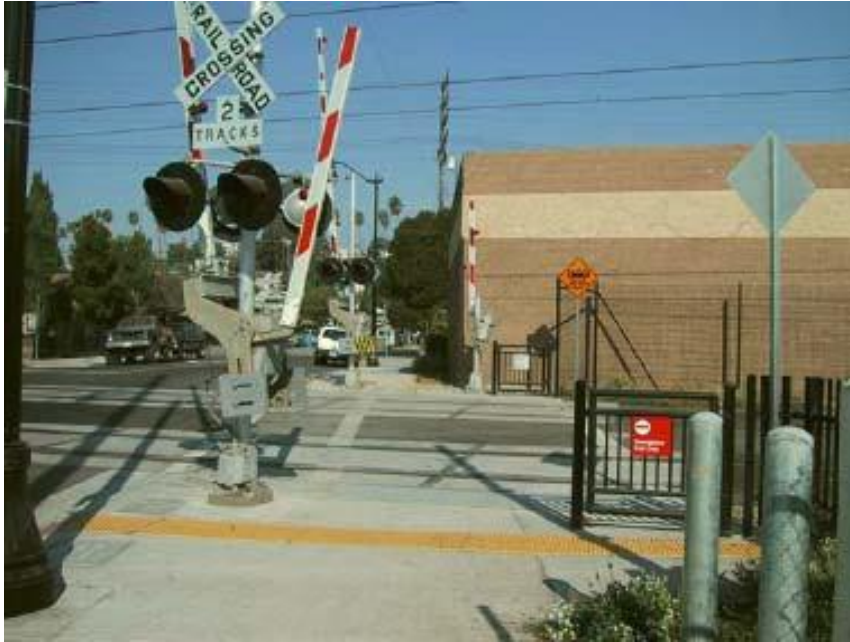
Figure 30. Standard railroad crossing flashing-light signals with gate arm, Gold Line LRT, Pasadena, CA
