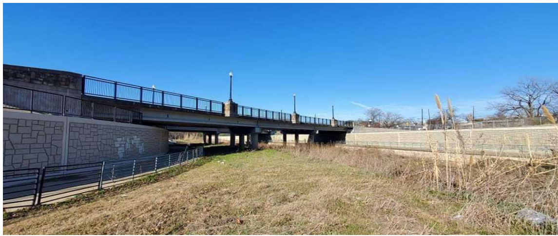
Figure 3. The photo of the first candidate (Bridge 1) on S Mesquite St. Arlington
