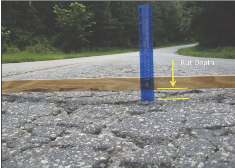
Figure 2.6 Pavement Rutting (Serigos et al., 2012)
