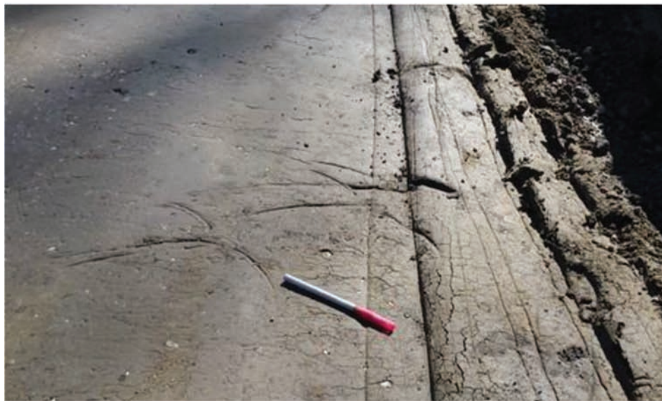
(b) Subgrade pumping
