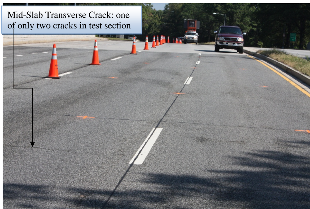
Figure 8: Condition of the Sawed and Sealed Section
