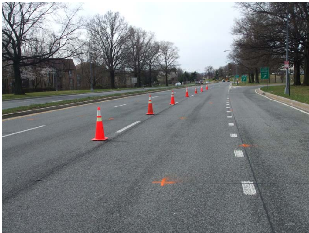
Figure 10: Condition of Treated Pavement Section
