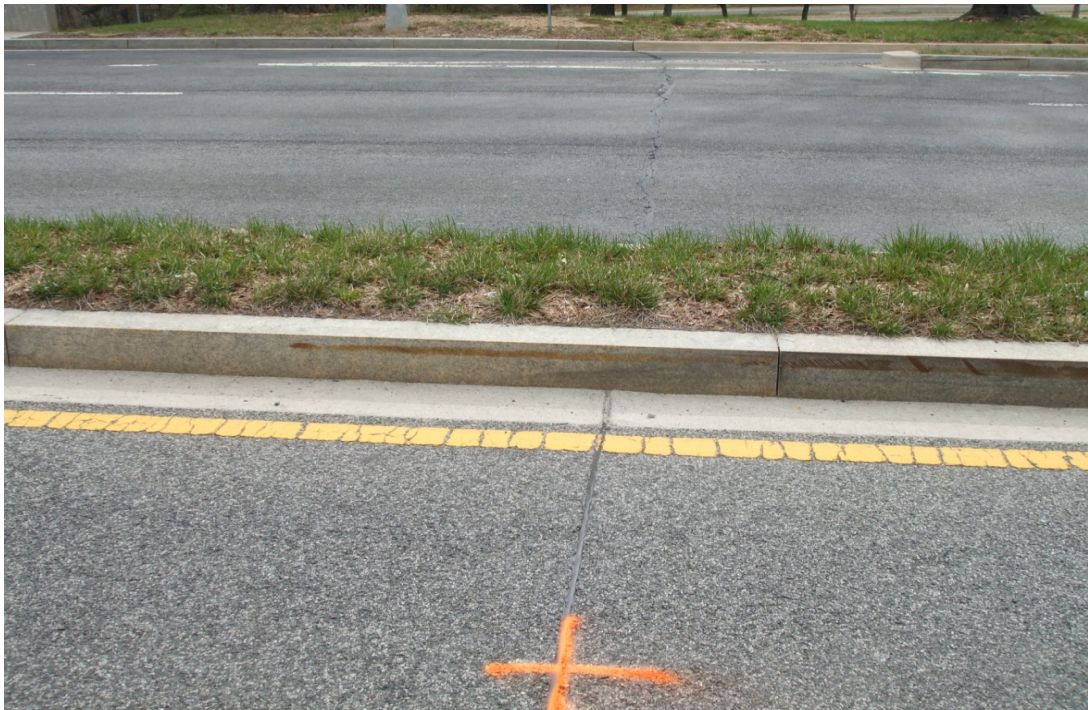
Figure 14: Typical Reflective Cracking Experienced at all Joint Locations in Untreated Pavement Section Adjacent to Corresponding Saw Cuts in Test Section.
