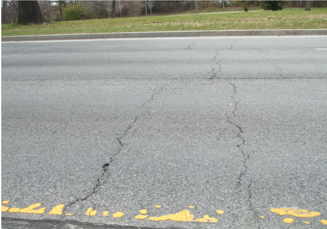
Figure 13: Major Cracking Area in the Untreated Pavement Section
