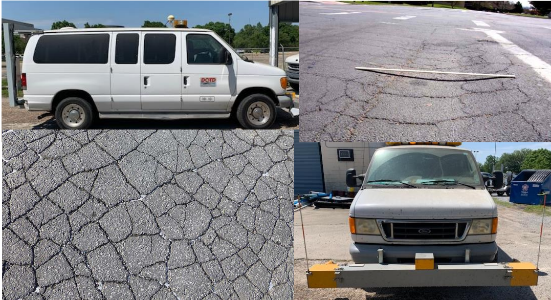
Figure 4. Automatic road analyzer (ARAN) and common distresses
