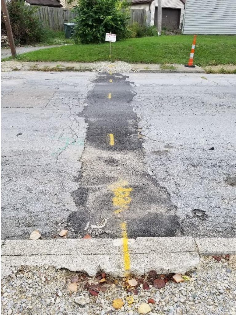
Figure 25 Example of temporary repair prior, City of Dayton.
