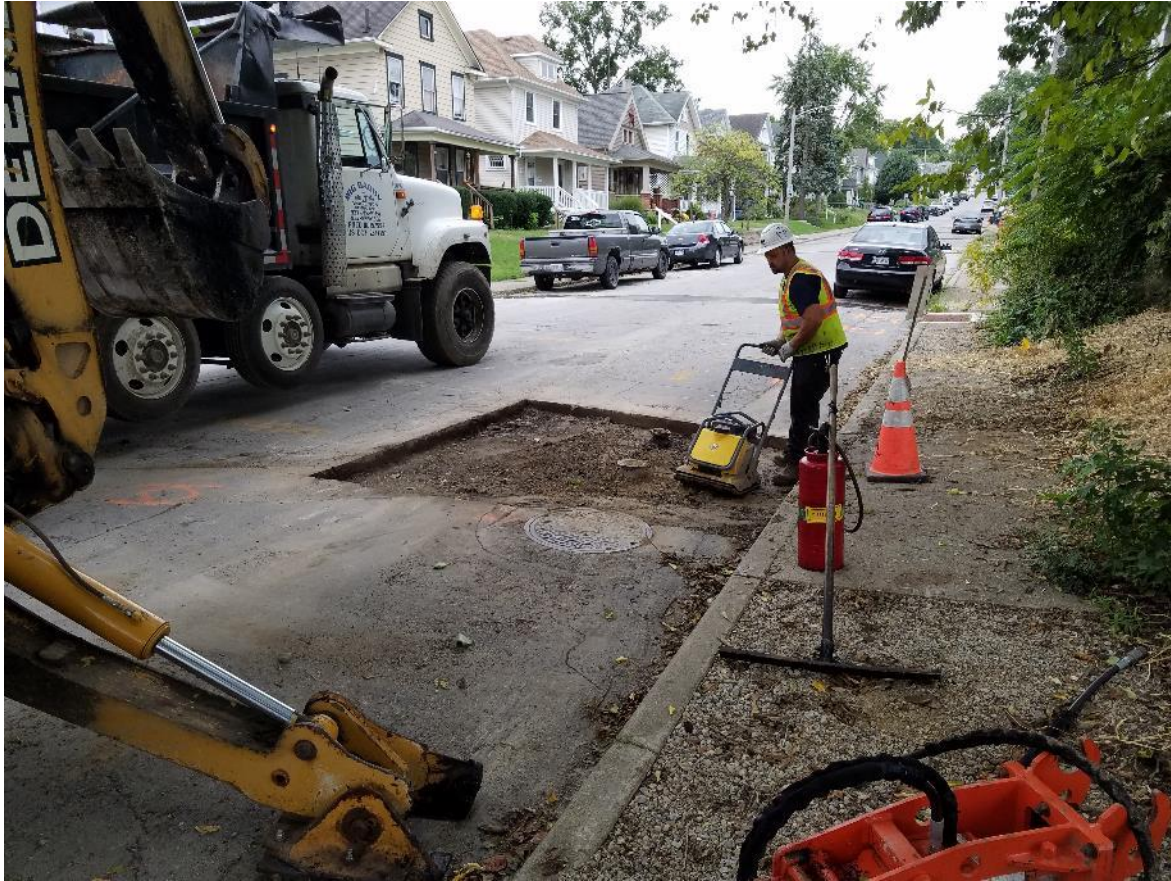
Figure 26 Example of granular base compaction during repair of open utility cut, City of Dayton.
