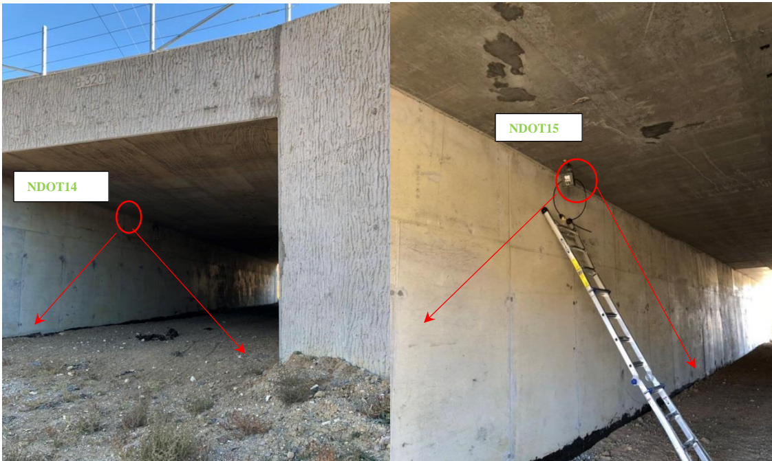
Figure 2-6 Locations and directions of the cameras at the north Wildlife Underpass on USA Parkway
