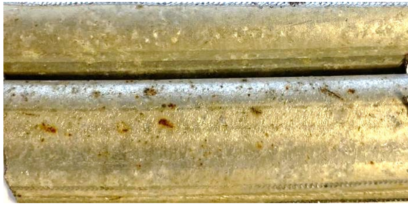
Figure 3.11. Preexisting corrosion in the form of pits around the corrugations and the lock-seam aluminized steel from Plant A.
