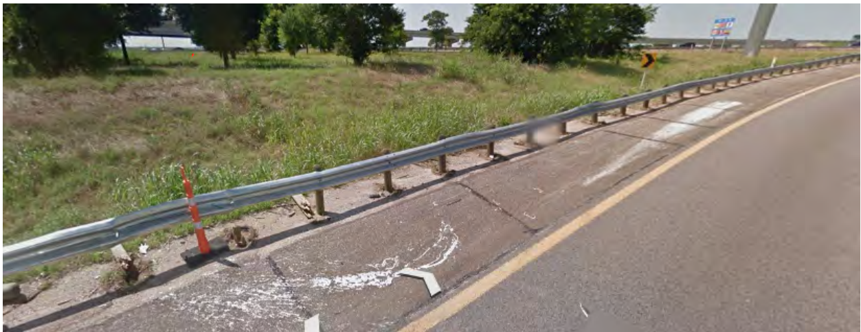
Crash Narrative 9: Intoxicated driver failed to drive in single lane and struck guardrail after failing to negotiate turn; incapacitating.
