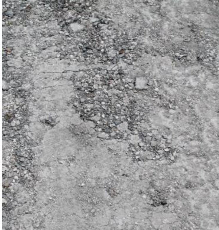
Figure 14 Typical base surface after the micro-cracking LA 599 Test Sections
