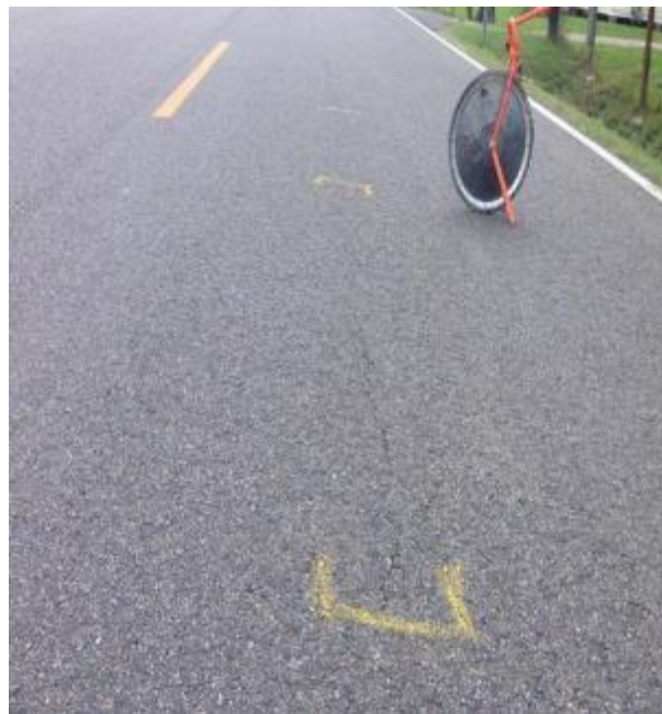
Figure 19 Crack survey on LA 1003
