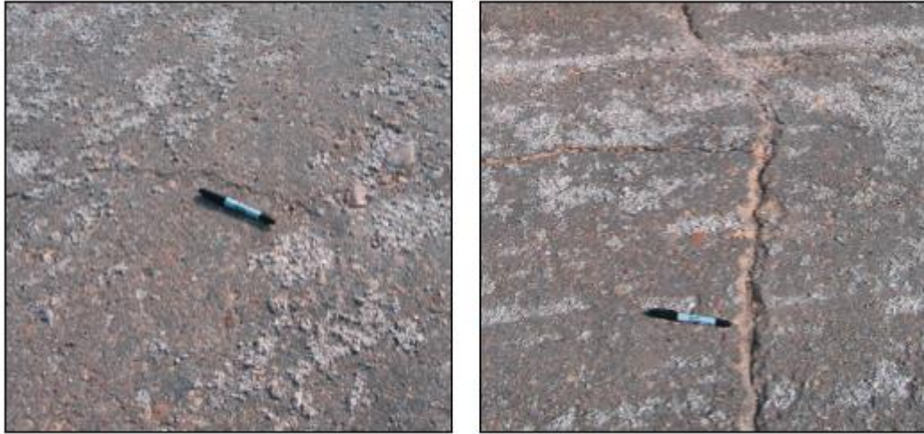
Figure 4 Shrinkage cracks in a micro-cracked section and an untreated section [8]
