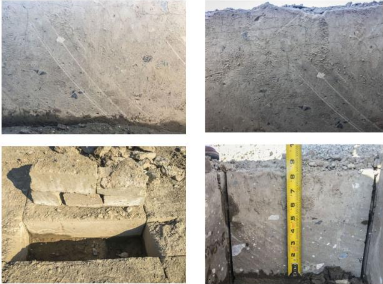
Figure 26 Saw-cut beam in Section III (micro-cracked section)
