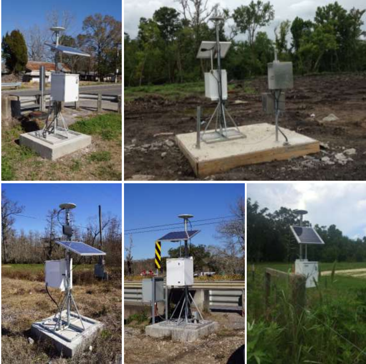
Figure 4 CORS 1-5 installations, in order from top left to bottom right
