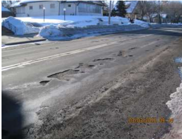
Figure 13 Stripping failure in HMA treated with chip seal [64]
