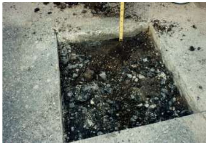
Figure 12 Pavement stripping in Pennsylvania [61]
