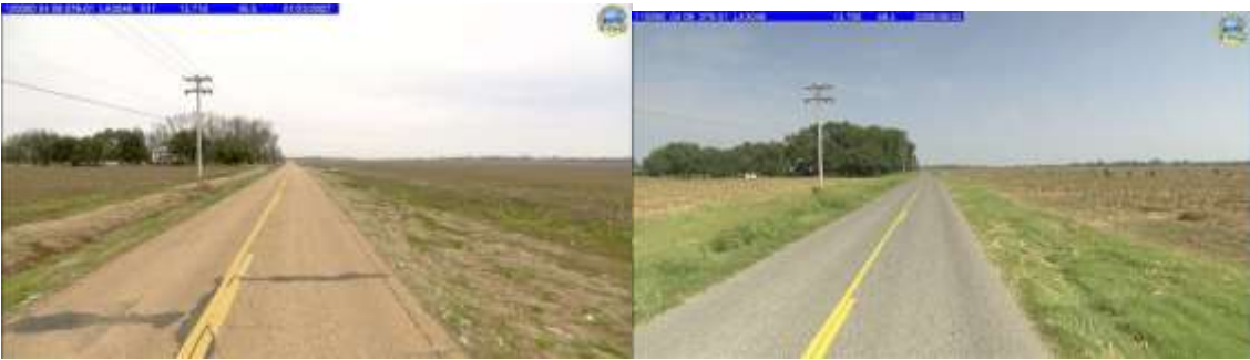
Figure 34 Pavement section before (left) and after (right) chip seal
