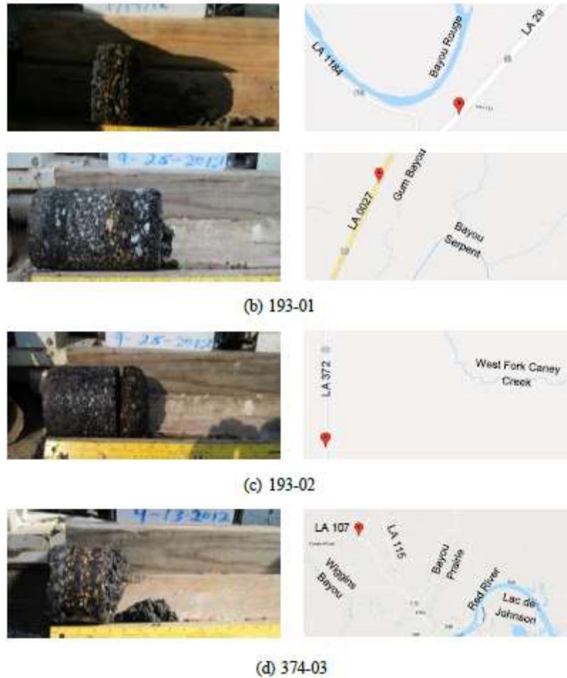
Figure 73 Moisture damaged sections with microsurfacing
