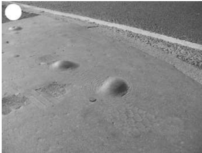
Figure 11 Blistering in asphalt pavements [58]
