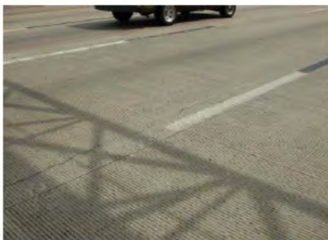
Longitudinal crack 1983 Experimental sections
