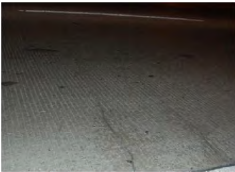
Typical transverse cracks
