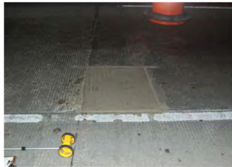
Small PCC patch
