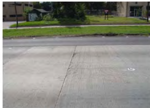
Patch with spall
