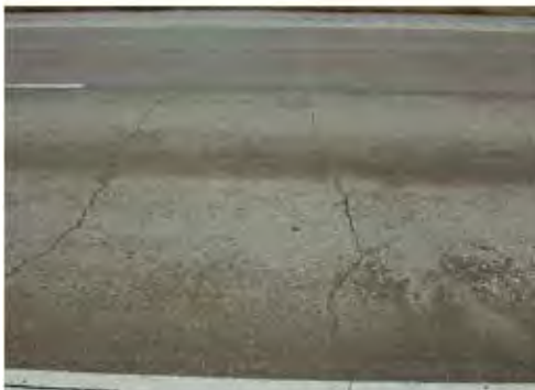
Picture 3 Transverse cracks
