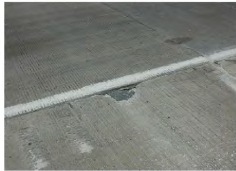
Shoulder joint damage
