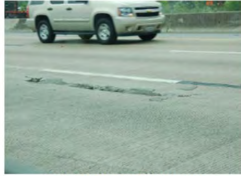
AC Patch, longitudinal cracks
