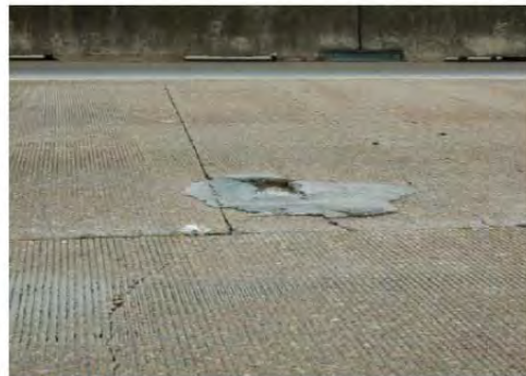
AC patch with failure
