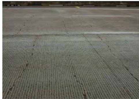
Closely spaced transverse cracks
