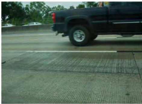
PCC patch with spall
