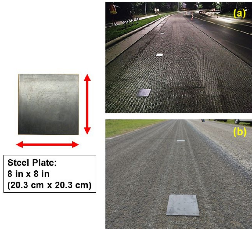
Figure 6. Steel plates placed on the roadway prior to emulsion application in (a) tack coat and (b) chip seal projects.
