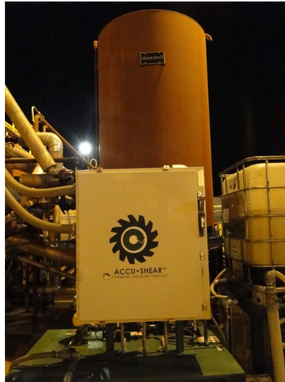
Figure 7 Accu-shear blending equipment
