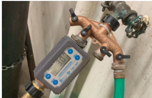
Figure 4.5: Flow Meter to Measure Inflow and Set Up Water Valve
