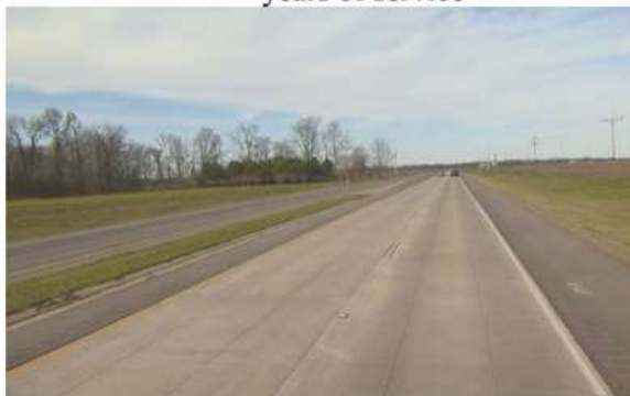
(c) UTW section on US65 after 9.4 years of service
