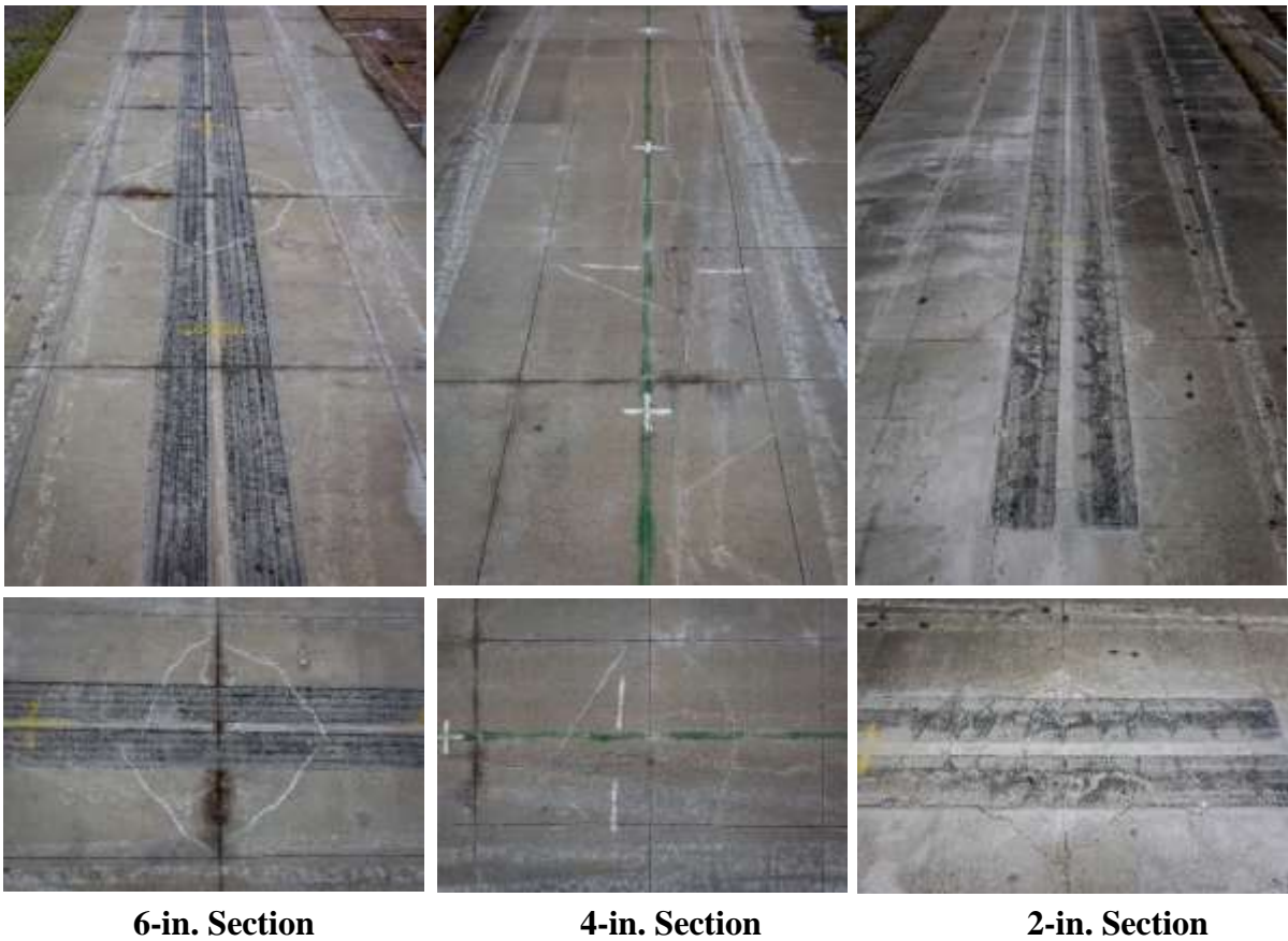
Figure 18 Visual distresses of BCOA pavement test sections
