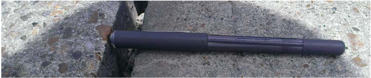
Figure 17 Faulting of adjacent pavement slabs for the 810-12 project slightly less than 1/4 in.
