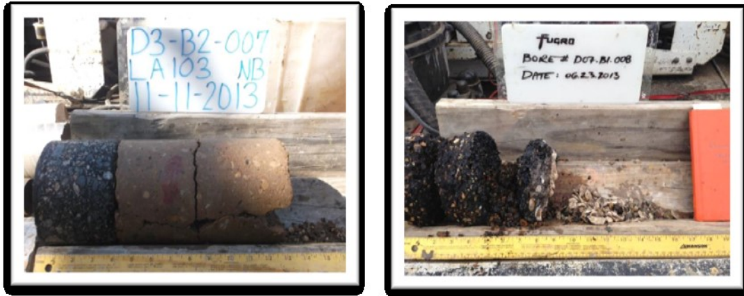
(a) Non-stripped pavement
