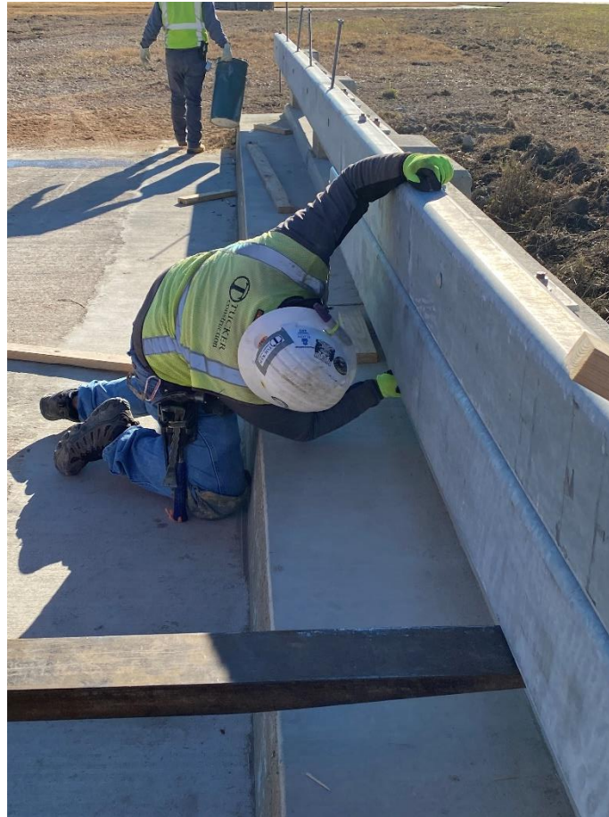
Figure 96. Installation of lower HSS10×4× \frac{3}{8} rail and bolting to top rail with \frac{5}{8} -in. diameter B7 threaded rods
