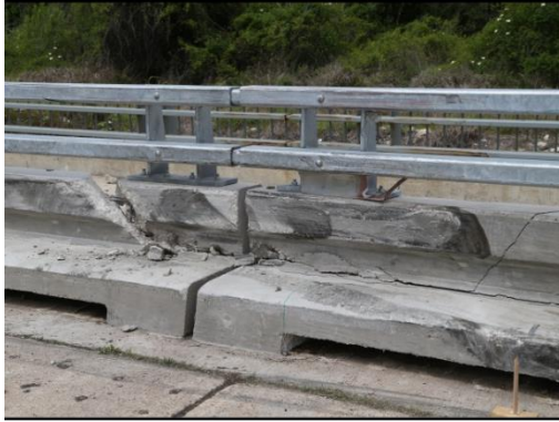
(a) Traffic side impact area damage test
