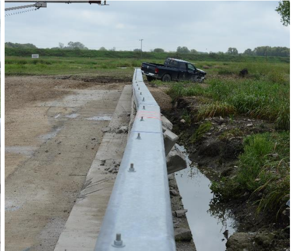
(b) Permanent deformation of bridge rail
