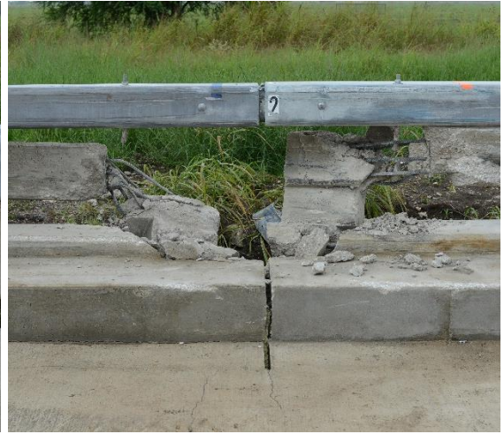
(b) Damage at joint 2
