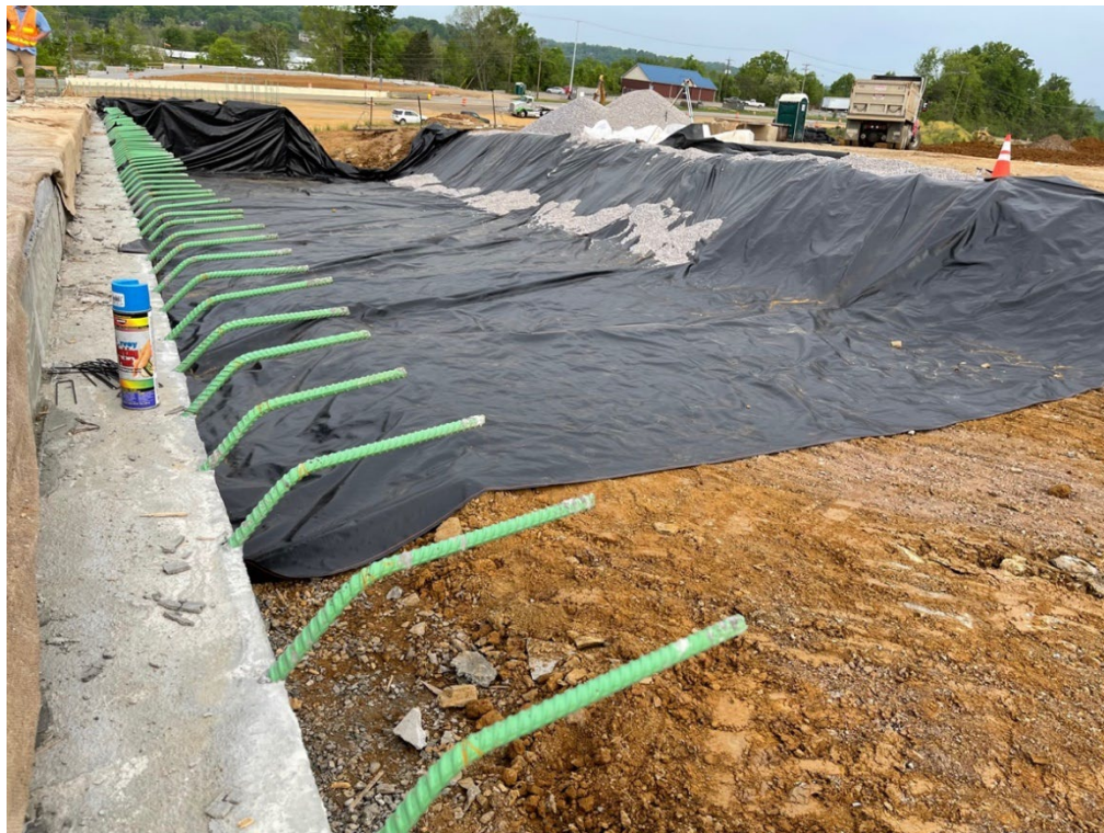
Figure 3-3. Propex GEOTEX-315ST Geotextile fabric laid at the bottom before placing the fill for the north approach slab.
