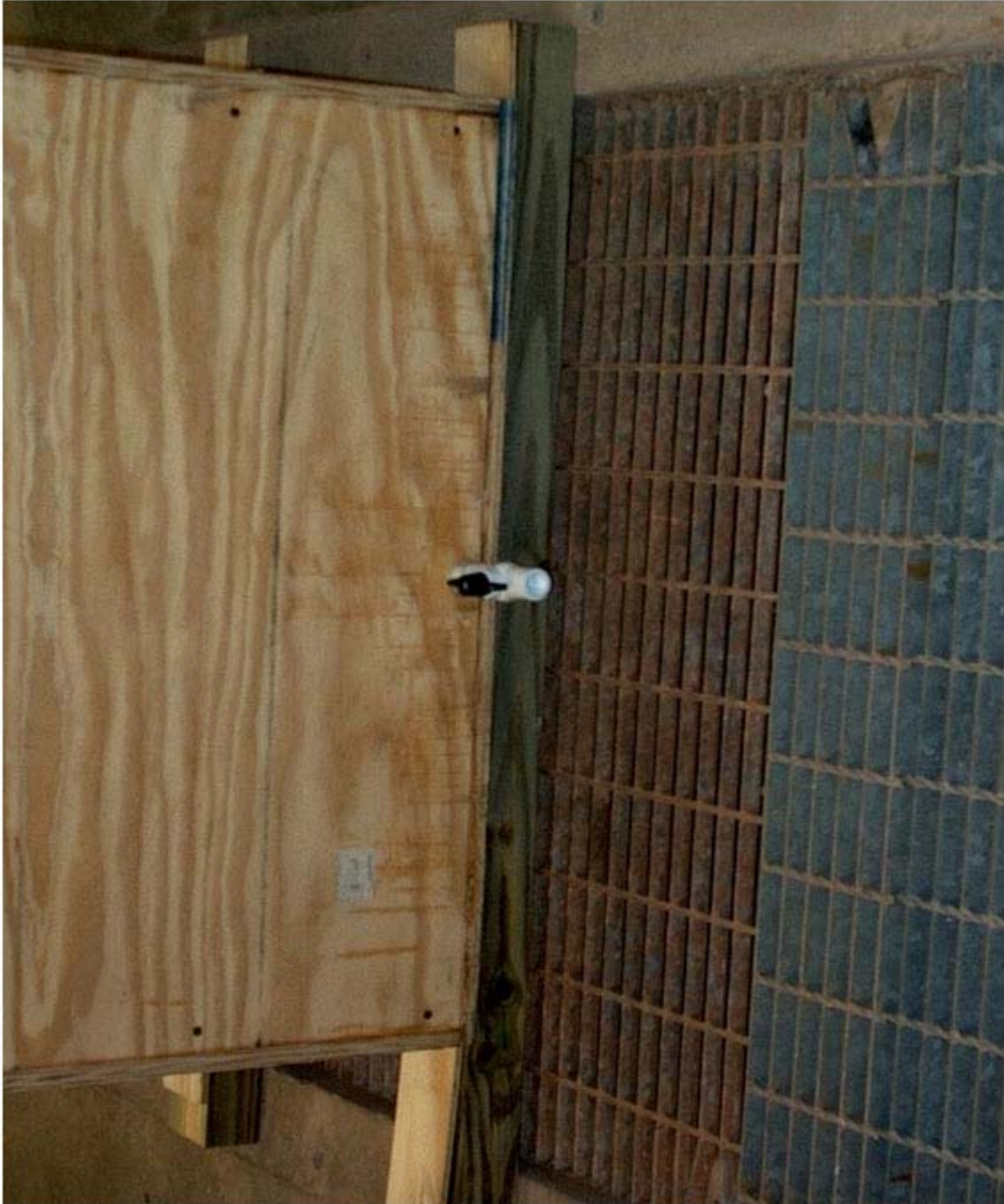
Figure 14. Drain valve to drain water from reservoir.
