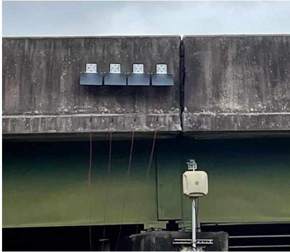
A. Solar panels mounted to the bridge.
