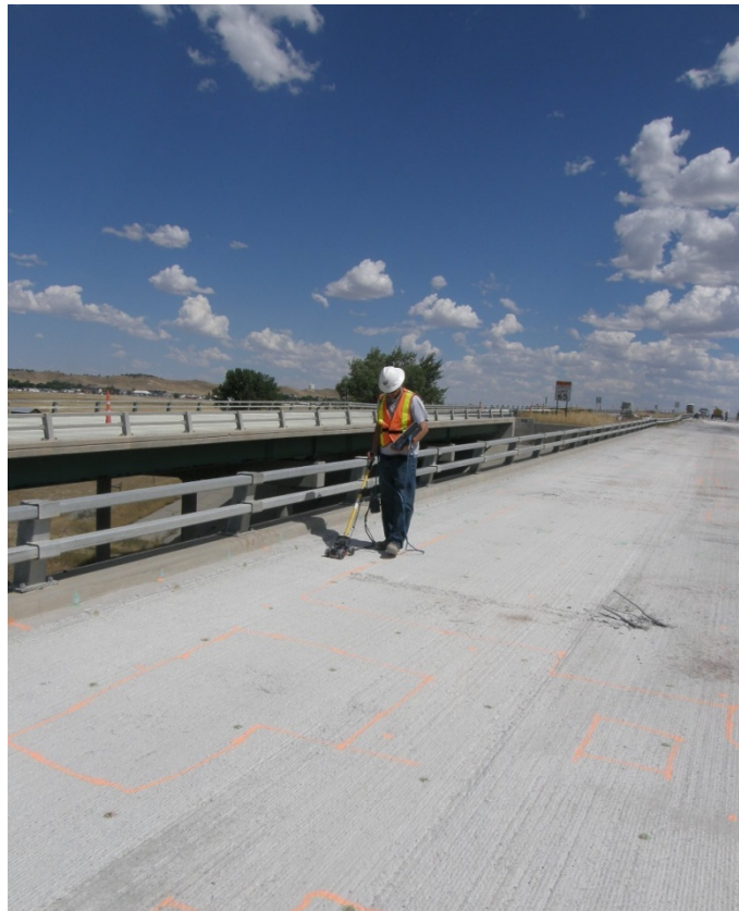
Figure 3 - GPR testing along the stripped surface of the bridge in Douglas Wyoming.
