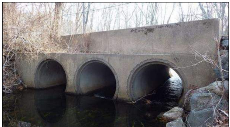
Bridge 06139, built in 1970, was formed from pre-cast concrete pipes; it carries Bloomingdale Road over Hunt's Brook in Waterford.
