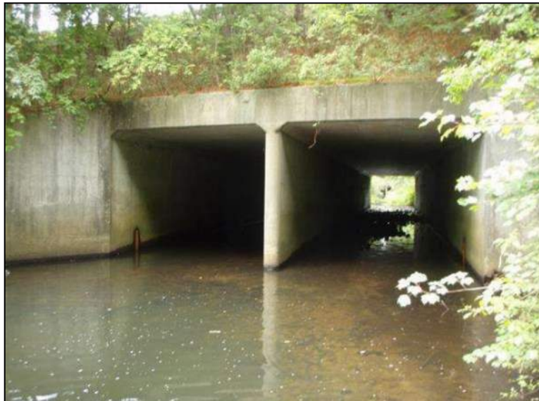
Bridge 02528, carrying Route 632 (North Frontage Road) over Sawmill Brook in Mansfield, was built in 1973 and is essentially identical to Bridge 00504.
