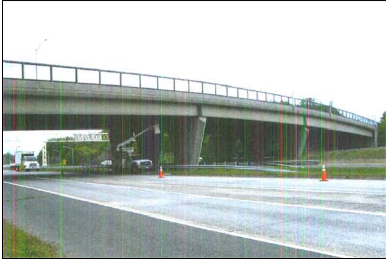
Many of the state's steel-beam bridges have multiple spans repeating the parallel-beam principle. This is Bridge 04248, Stanley Street over Route 9, New Britain, built in 1977.
