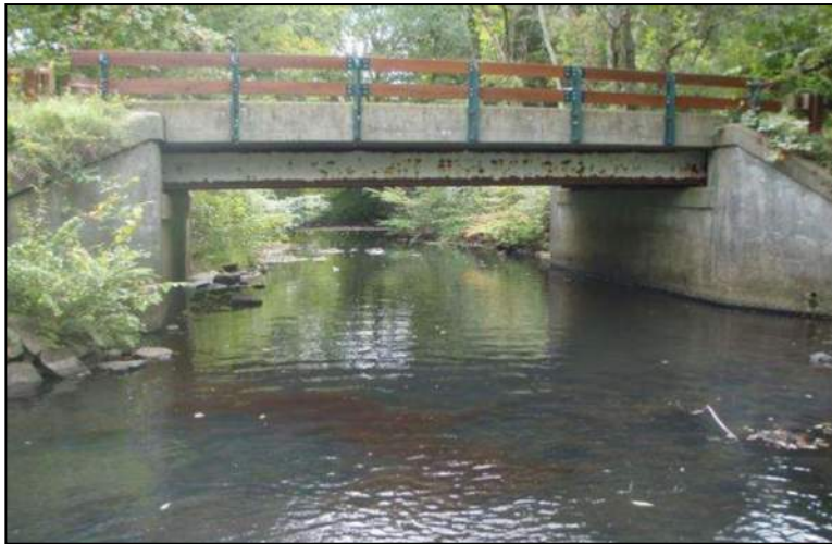
Bridge 04694 is a steel-beam structure built in 1946. It carries North Bigelow Road over the Little River in Hampton.
