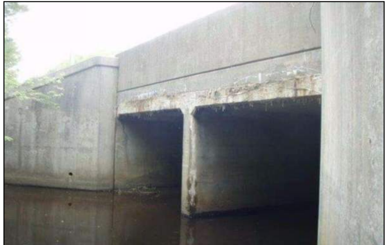
Bridge 00504, carrying Route 6 over Quanduck Brook in Killingly, is a cast-in-place dual box-culvert bridge built in 1946.
