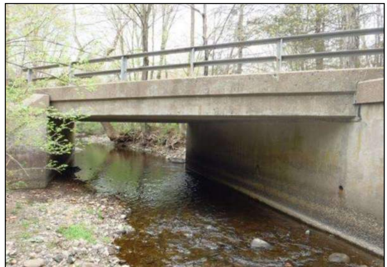
Bridge 03706 is another typical concrete-slab Post-World War II bridge. Built in 1963, it carries Plumtrees Road over East Swamp Brook in Bethel.
