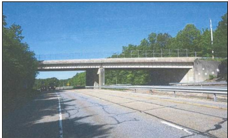
Some of the state's steel-beam bridges use girders with welded-on vertical stiffeners rather than simple rolled I-beams, such as Bridge 00306 (1958), which carries Squaw Rock Road over Route 695 in Killingly.
