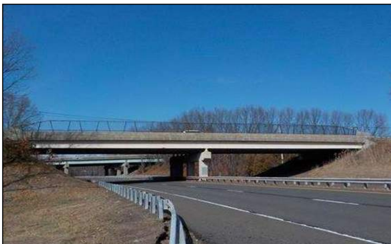
Some of the state's multiple-span steel-beam structures employ the continuous-beam principle, in which there is no break in the beam over the intermediate piers. This allows a smaller cross-section for the same load-bearing capacity. This example is Bridge 00387 (1950), carrying Route 94 over Route 2 in Glastonbury.
