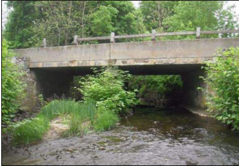
Bridge 01589 is a typical concrete-slab bridge of the Post World War II period. It dates from 1947 and carries Route 318 over Morgan Brook in Barkhamsted.
