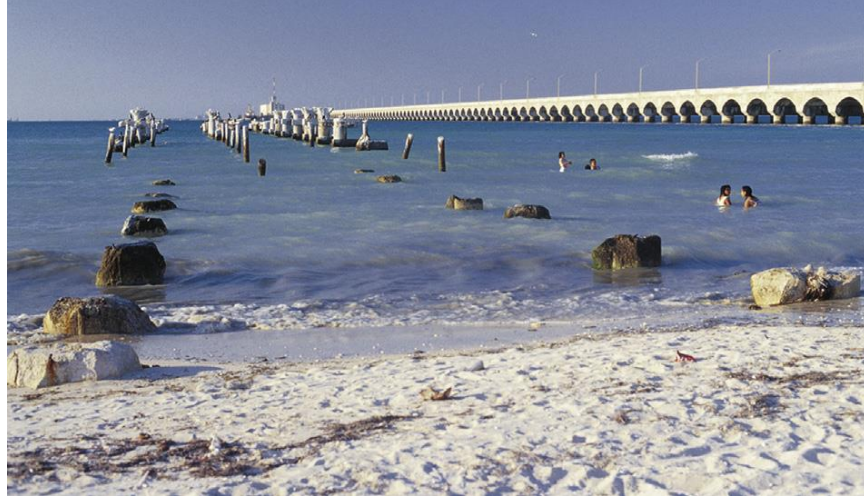
Figure 3.4: Two piers built in Progreso, Mexico. Far right, pier built with stainless steel, completed in 1941. Left, remains of pier built with black steel 30 years later (Hansson 2016)
