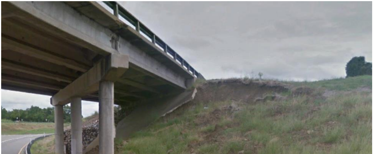
Figure 9.1 Slope failure at the intersection of SE Loop 286 and Clarksville St, Paris, Texas
