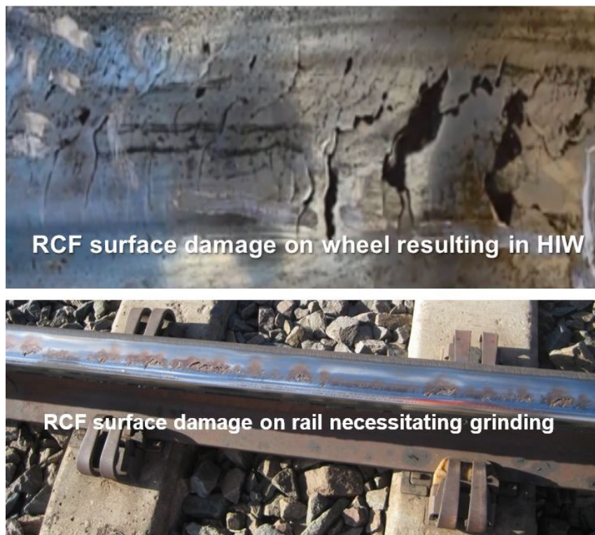
Figure 1. Wheel and rail RCF
