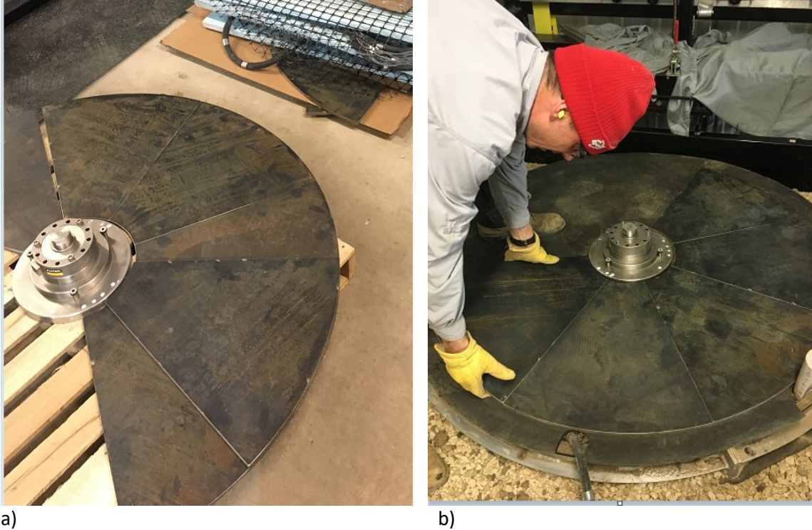
Figure 18. Steel surface plate installation: a) set first layer of steel plates and b) set the second layer of steel plates
