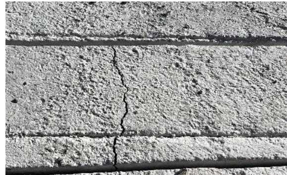
Figure 6 - PR concrete with embedded cracked during the pull testing.
