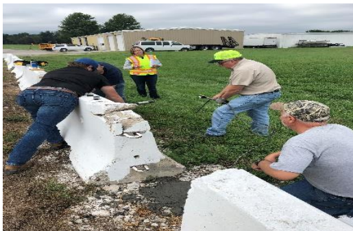
Figure 2 - Physical Tests technicians perform the pull-out test. Tie-bars were inserted into concrete barriers to determine the strength of non-shrink grout.
