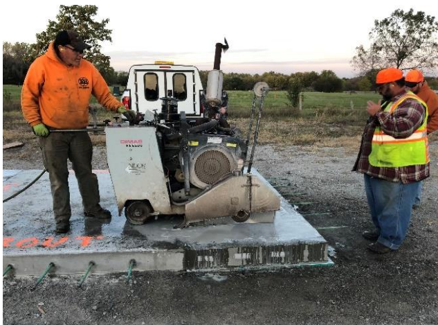
Figure 4 - The Salt Valley maintenance crew sawed through the thickness of the PR slab. Foam inserts prevented cutting into the 47BD slab.
