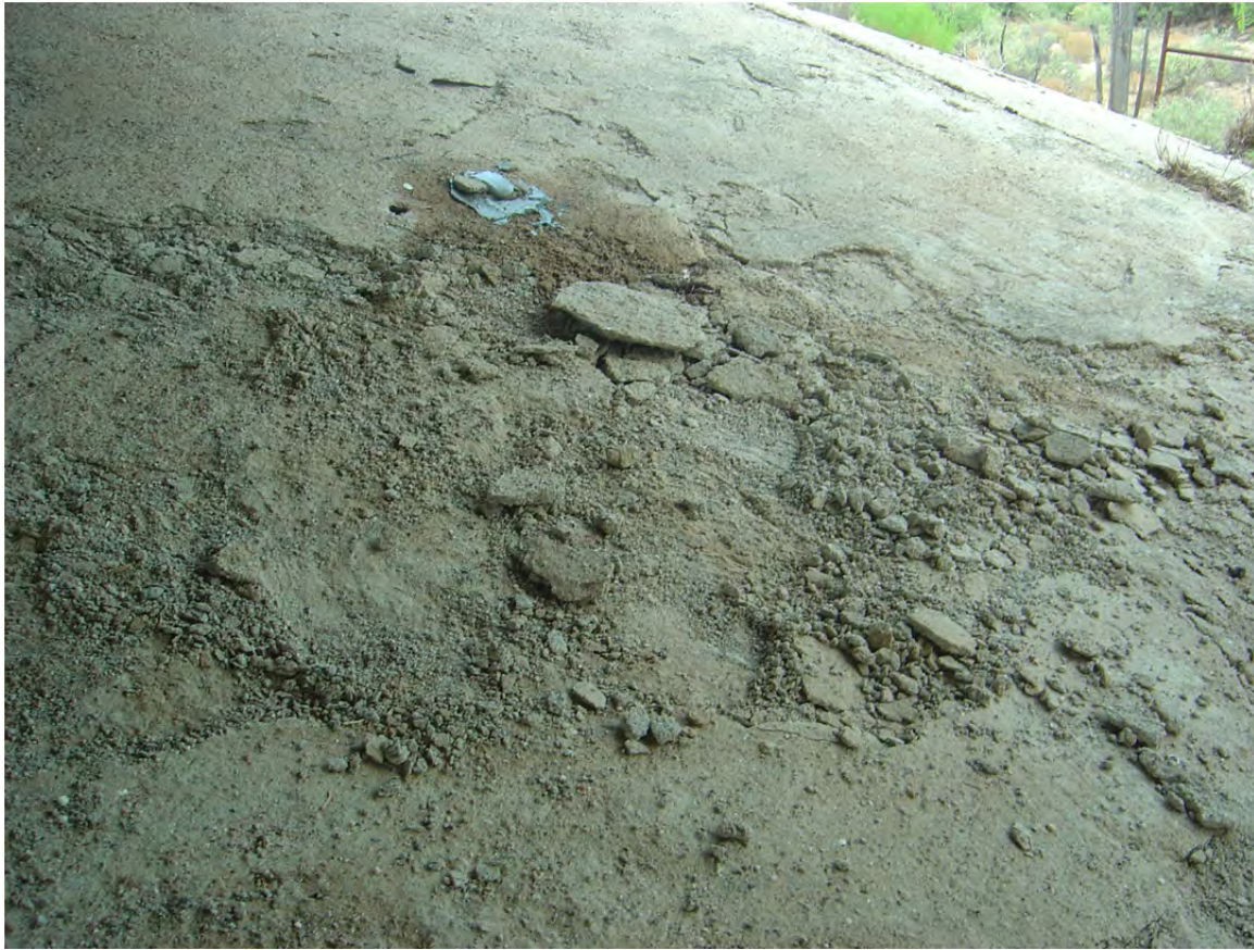
Figure 7.9: Riprap deterioration at Site 31 in the El Paso District
