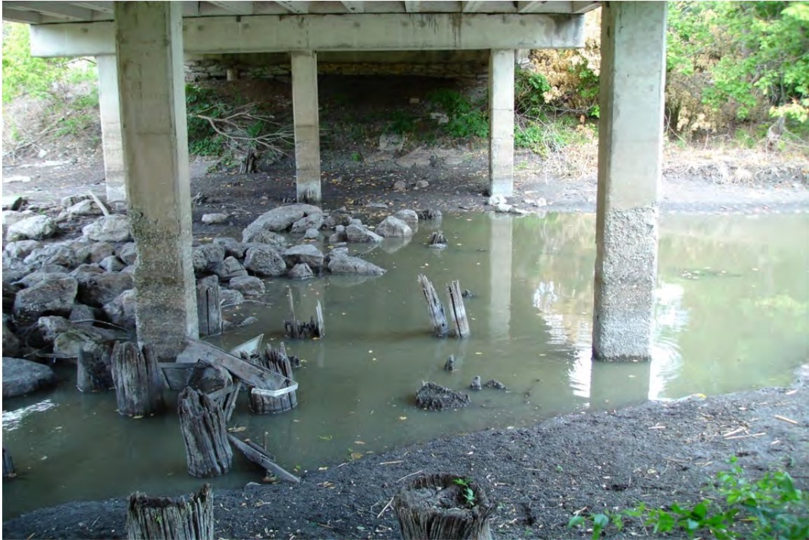
Figure 7.7: Deteriorated concrete columns from a bridge in the Paris District
