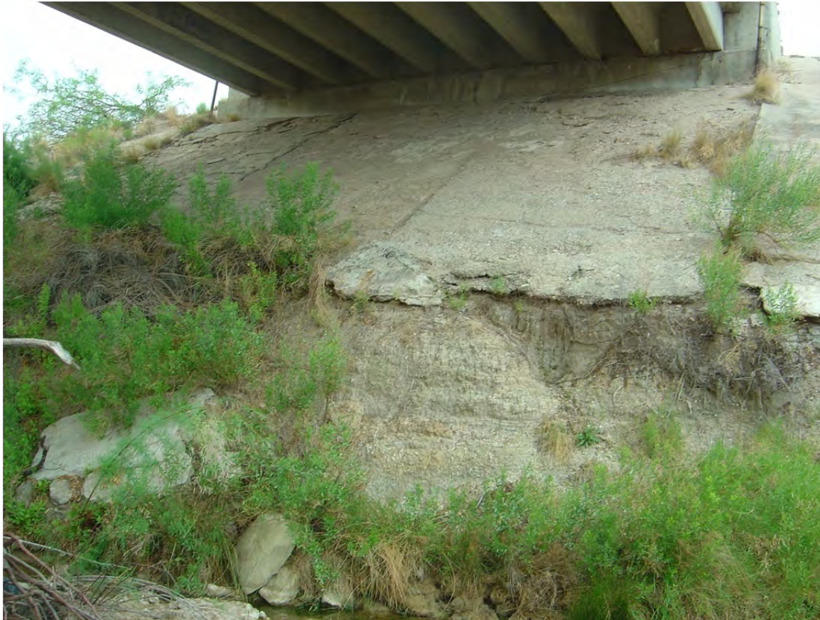
Figure 7.10: Deteriorated Riprap at Site 32 located on FM 652 in the El Paso District
