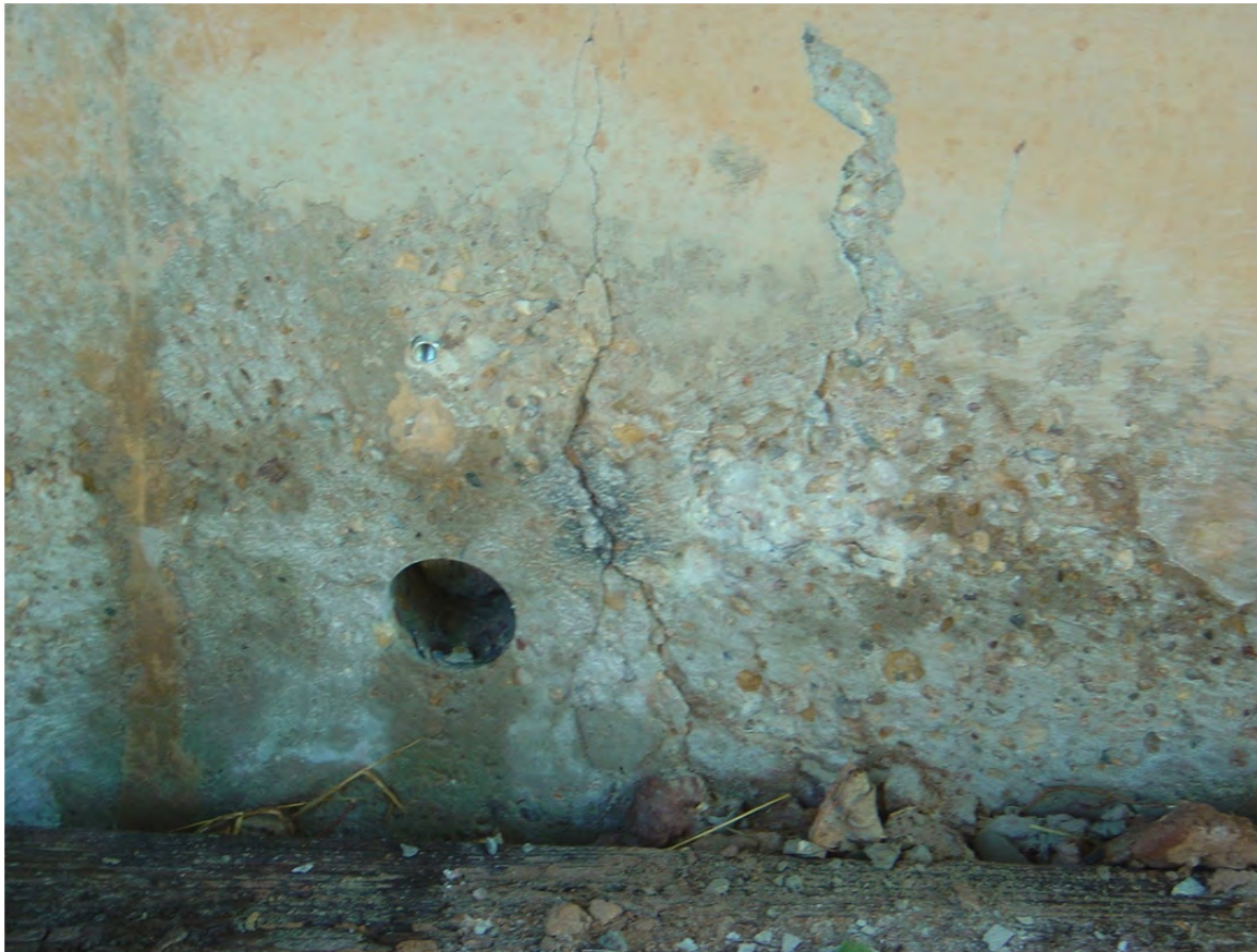
Figure 7.3: Damage to the lower part of a wall below US 83 in Childress District
