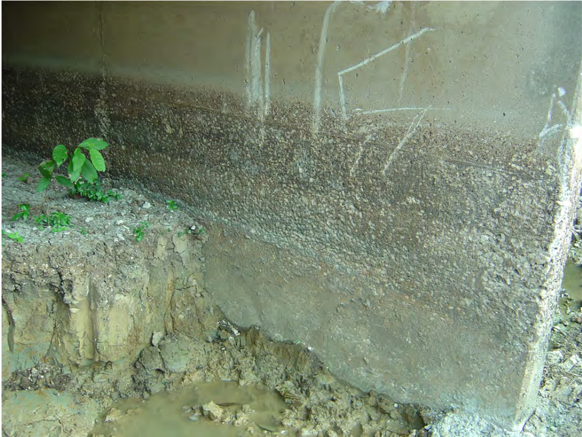
Figure 7.6: Deterioration of a culvert above the soil level, with no deterioration visible below the level of the soil (after excavation)
