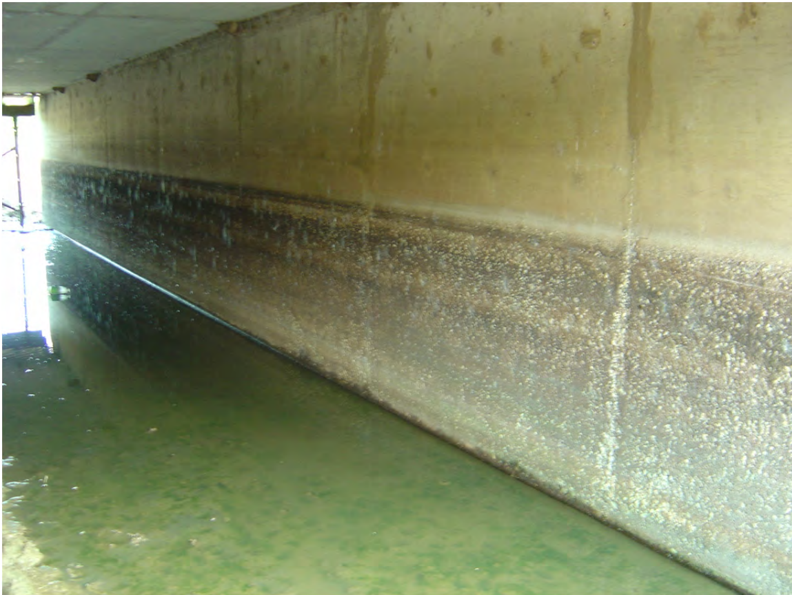
Figure 7.5: Deterioration commonly found in culverts in the Paris District. The distress begins near the base of the culvert and continues up the side, likely in line with the highest level of water.
