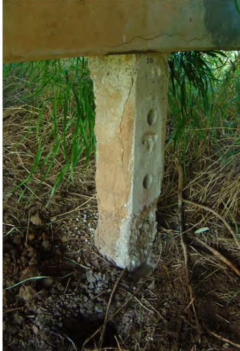
Figure 7.4: Damage to a bridge column on FM 2278, south of Childress, Texas
