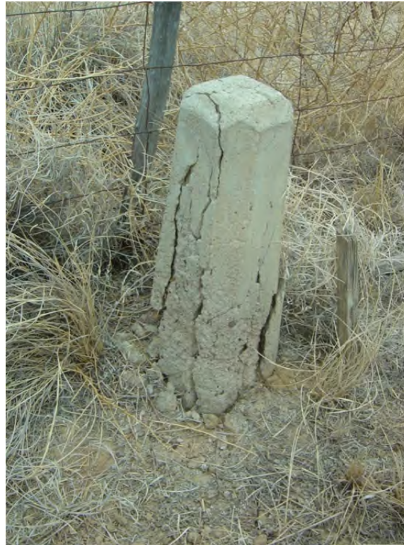
Figure 7.11: ROW marker deteriorating in West Texas.
