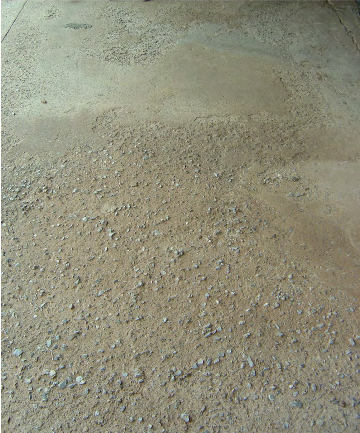
Figure 7.8: Riprap deterioration occurring on the embankment below a bridge
