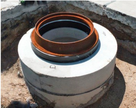
Figure 4. Concrete adjustment rings.
