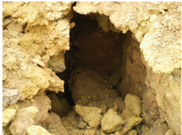
Figure 2.4 Close-up view of a sinkhole near Salem Bypass in Washington County, Indiana (T. Colglazier & N. Z. Siddiki, personal communication, November 14, 2017).
