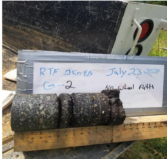
Figure 4. Core Showing Delamination in Multiple Layers and Moisture Damage at Bottom Layer (Rte. 250 EB, Richmond District)
