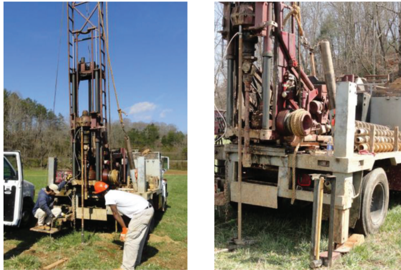
Figure 1.13 Advancement of penetrometer and extension rods using a conventional drill rig at a site located near Franklin, NC, USA.
