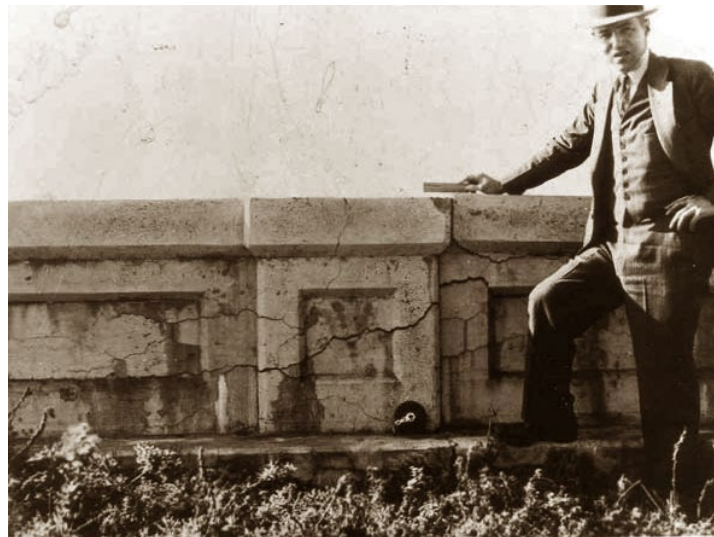
Figure 2.1 "Thomas Stanton of the California State Division of Highways and a Bridge Parapet Wall Showing Signs of Damage due to Alkali-Silica Reaction" (Thomas, 2013).
