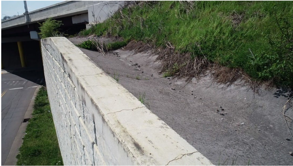
Figure A. 3 Cracks observed on top of the wall, clear drainage path on top of the wall
