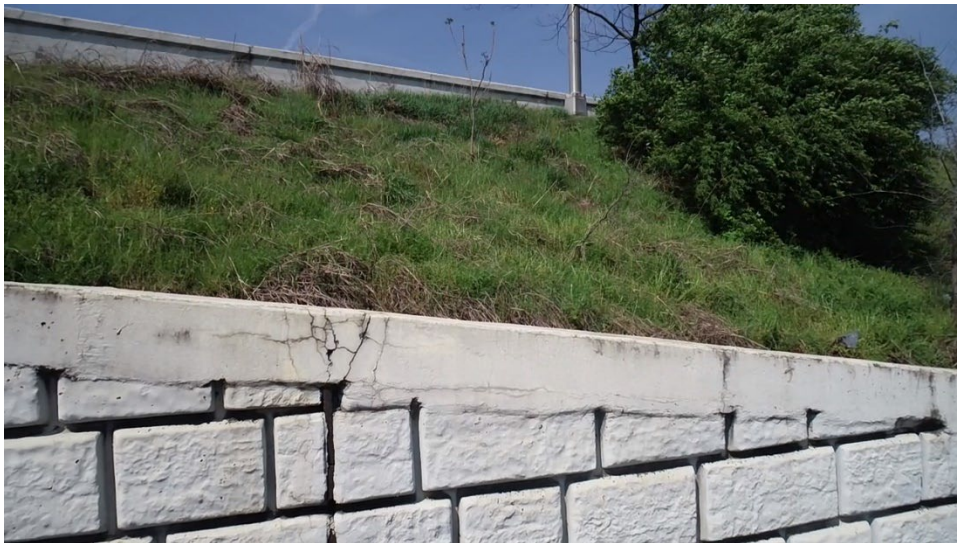
Figure A. 2 Cracks observed on top of the wall
