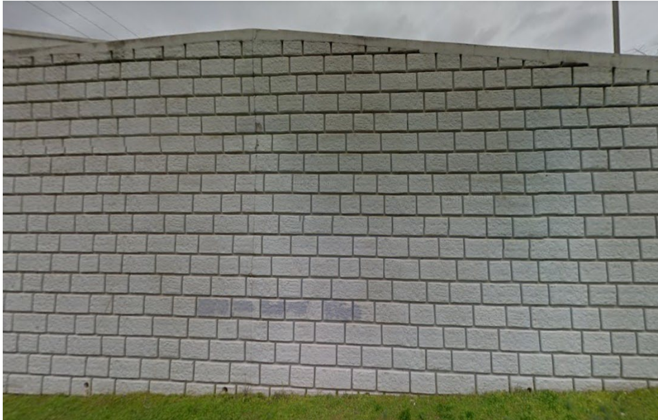
Figure A. 1 Vertical crack on wall facing
