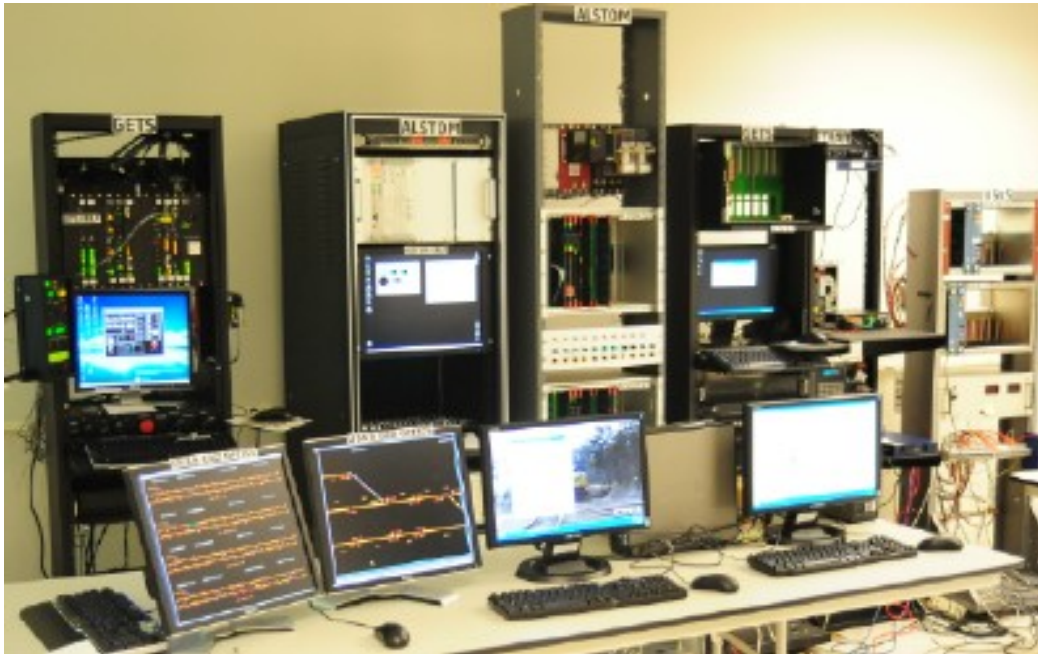
Figure 8. ICBS project equipment located at the Critical Link facility
