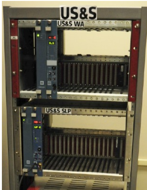
Figure 15. The Anslaldo-STS (US&S) equipment. Both their SLP and WA are based on their MicroLok® product line
