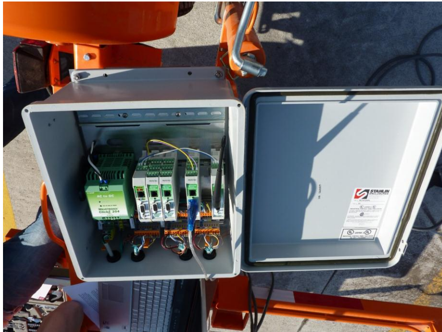
Figure 3.12 Portable sensor pole cabinet
